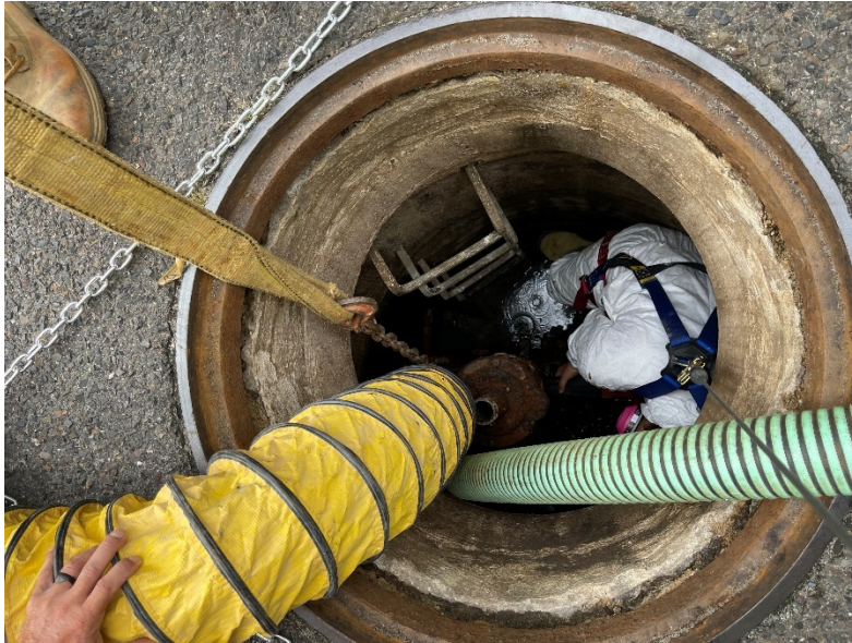
Replacing an Air Release Valve on one of the Authority's Secondary Force Mains
