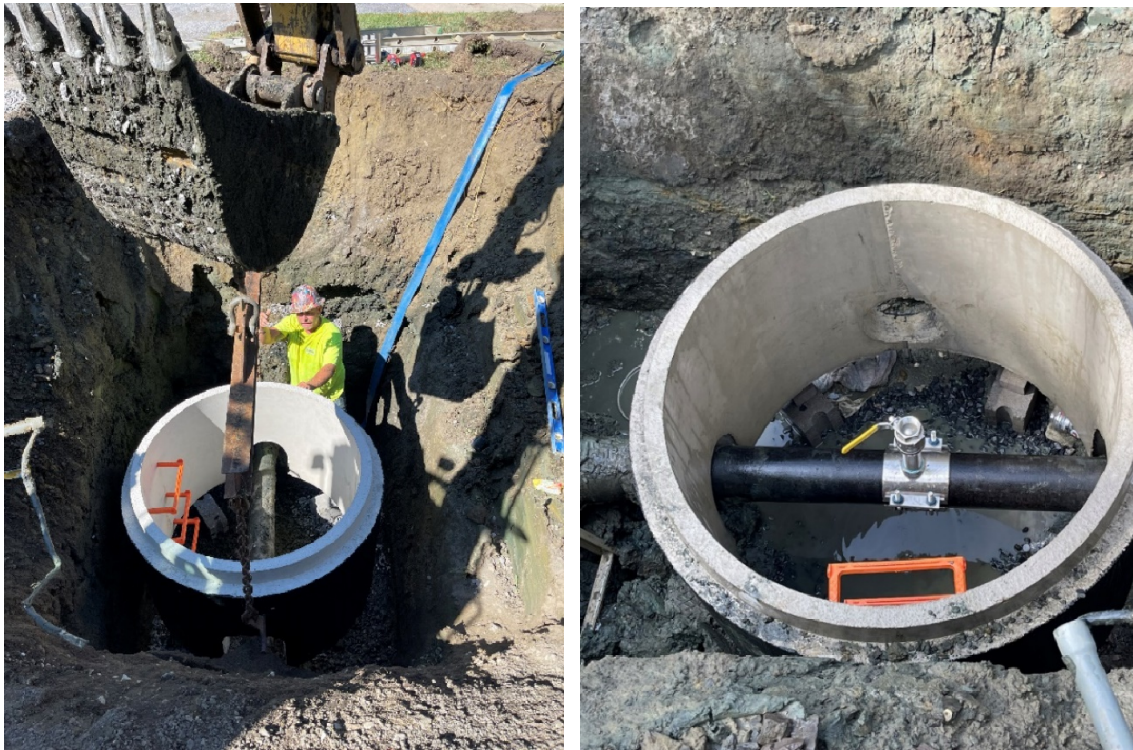
Installation of a New Air Release Valve on the 40-year old Tricia Meadows Force Main along Mount Laurel Road
