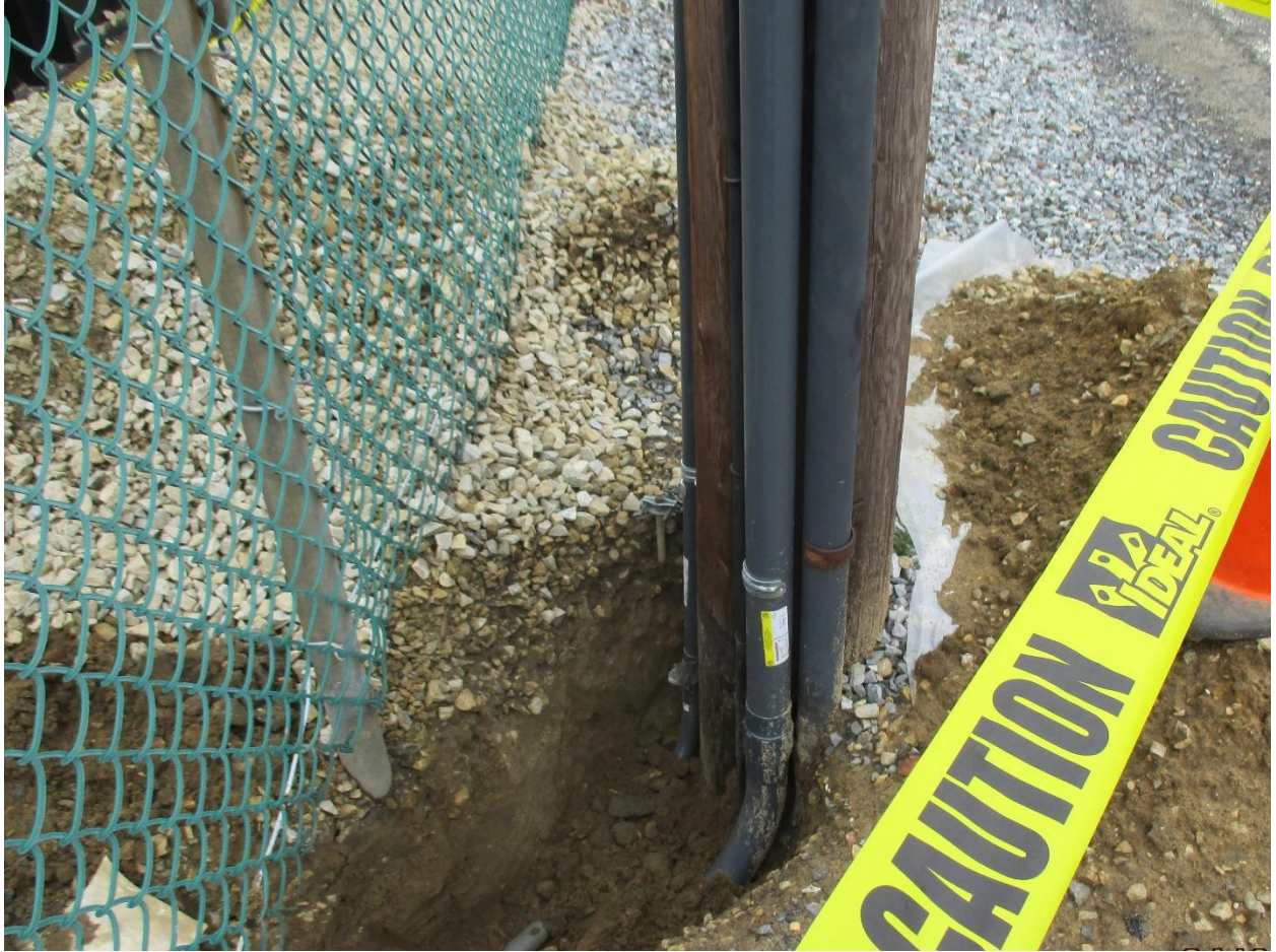
New conduit at Turnpike Pump Station
