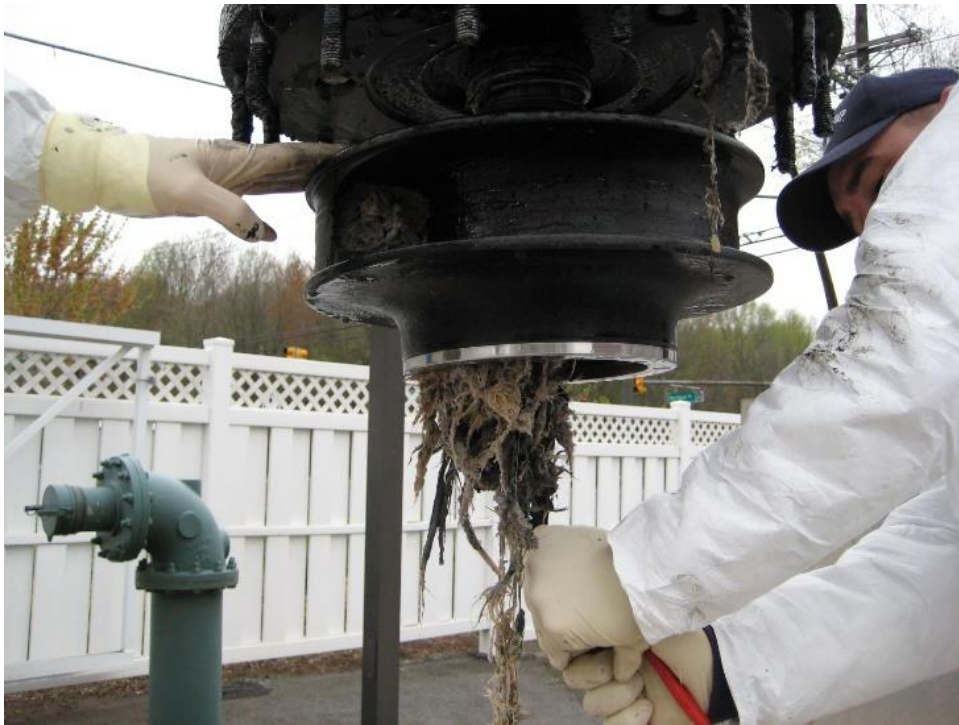
Clearing “Flushable” Wipes from one of 3 Clogged Pumps at Larchmont PS
