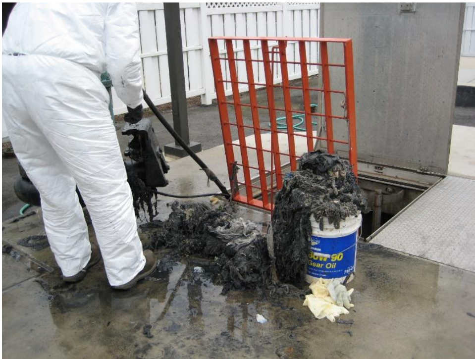
MUA Employee Removing “Flushable” Wipes from Larchmont PS
