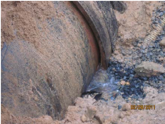
The leak found after excavation
