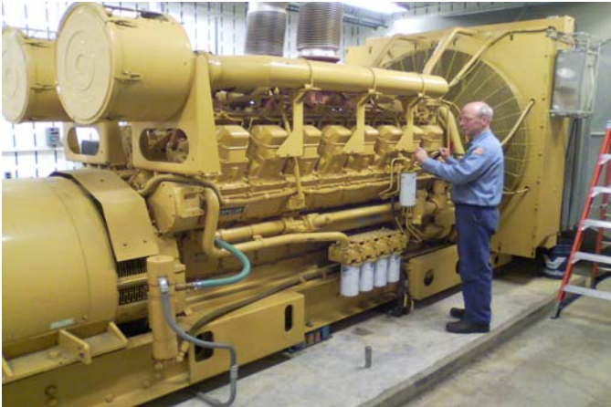
Stand-By Generator for Hartford Road WPCF
