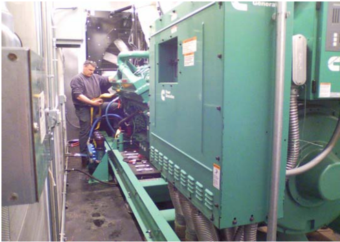
Stand-By Generator for Elbo Lane WTP
