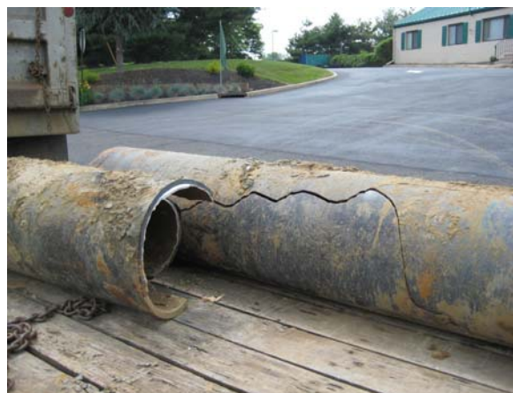
Cracked main, trucking for forensic analysis
